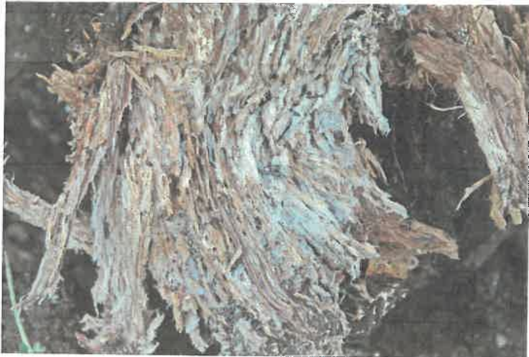
Advanced decay leaving white stringy, spongy wood.
