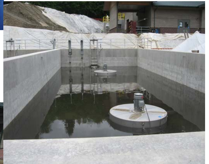
Anoxic Basins Mixers Installed
